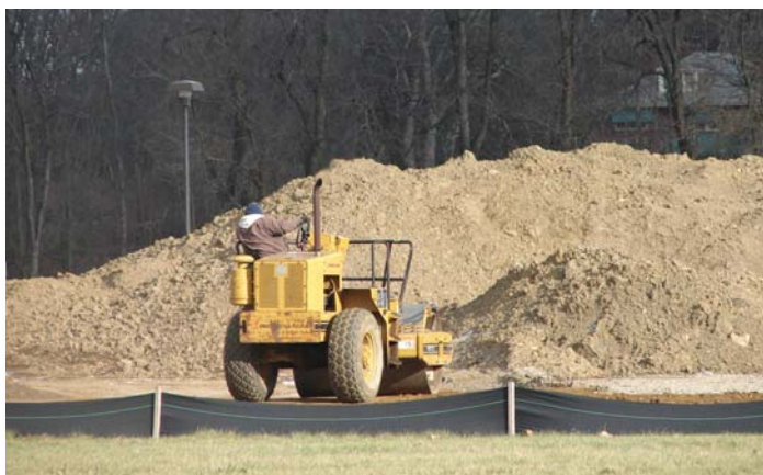
Construction continues on the future John L. and Christine Warner Library and Student Center.
